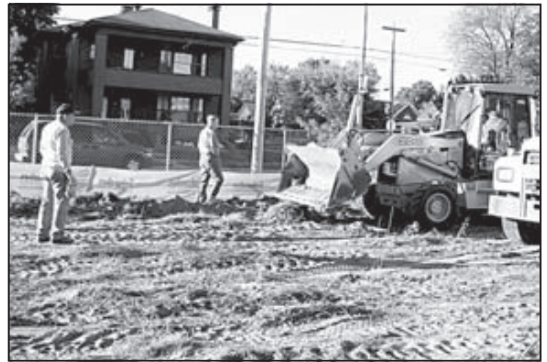
Darrell Howard and Bobby Beavins watch as Phillip McCarthy finishes digging up the first truckload of dirt. Submitted Photo
